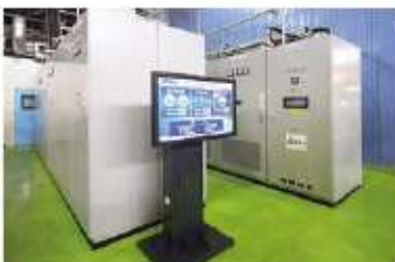
Power recovery system
