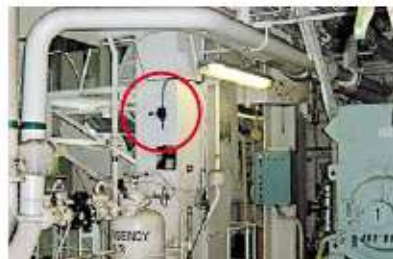
Beside generator engine
