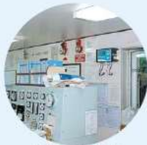
Engine control room
