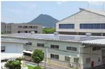
Photovoltaic power generation
