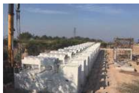
Gas generator set power plant project in Iran
