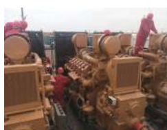
Kazakhstan Gas Coupling set Unit Project
