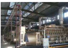
Biogas generator set power plant in Nanjing
