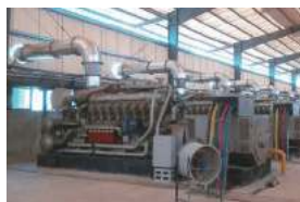
Gas generator set power plant project in Ghana
