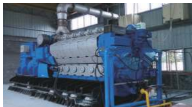
Gas generator set power plant in Bengal
