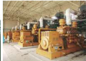
Gas generator set power plant project in Nigeria
