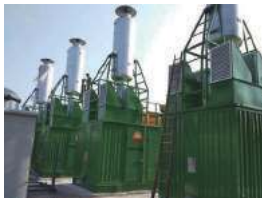
Gas generator set power plant project in Russia
