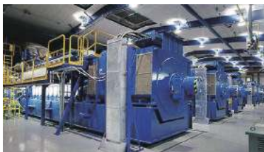
Gas generator set power plant in Saudi Arabia
