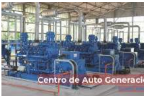
Gas generator set power plant project in Columbia
