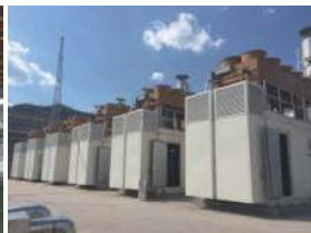
The coal mine gas genset power plant project in Ningxia
