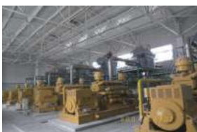
Biogas generator set power plant in Thailand
