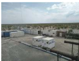
Oilfield associated gas generator set project in Kazakhstan
