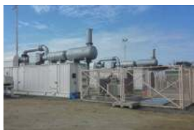
Gas generator set power plant project in Peru
